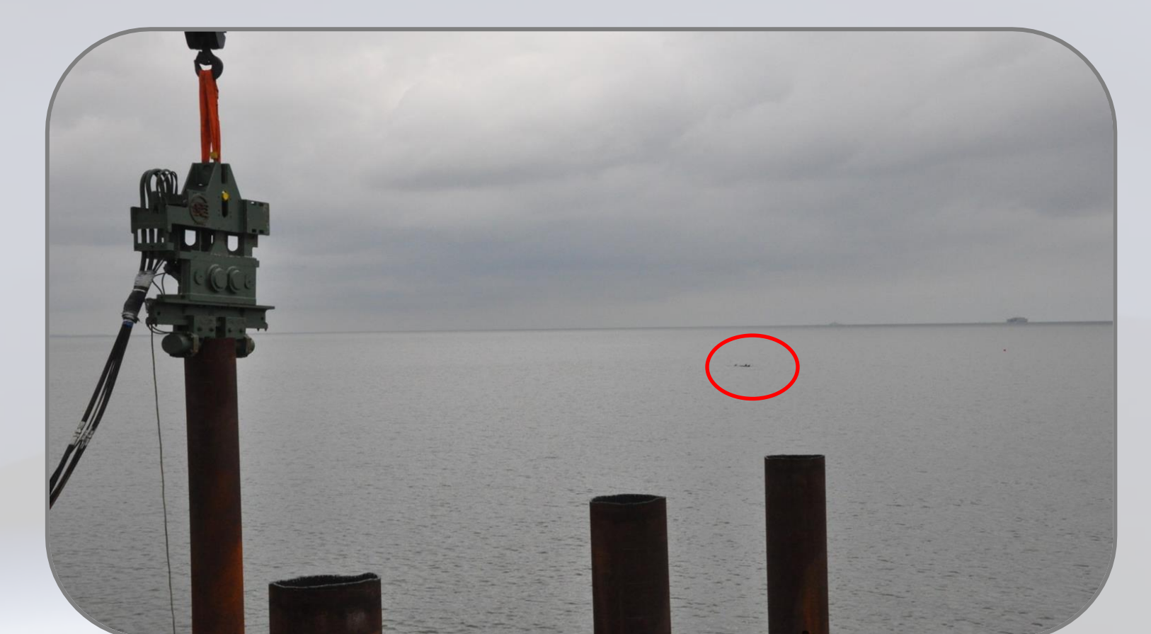
Fig. 5. Marine mammals ( Tursiops truncatus ) sighted during vibratory extraction of 24" steel pipe piles at JEB Little Creek.
